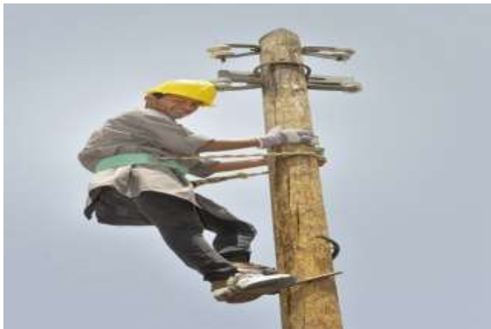
Student Emad Abu Holli climbs a utility pole during a class on electrical wiring at the Vocational Training Center in Khan Yunis, Gaza
